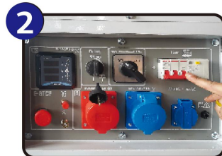
TURN OFF THE CIRCUIT BREAKER.
