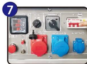
TURN ON THE CIRCUIT BREAKER.
